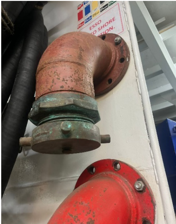
2 x 8" manifolds to connect to 2 x risers on main deck, in turn connected to 2 x 6" hoses from the terminal
