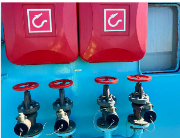
8 x 2.5" hose manifolds, 4 port and 4 starboard on the main deck
