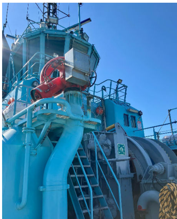
2 x 2000m 3 /hr combined foam & water monitors, one port, one starboard aft
