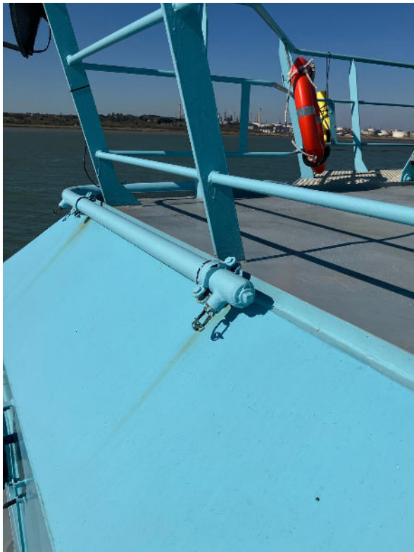
Accommodation drench system
