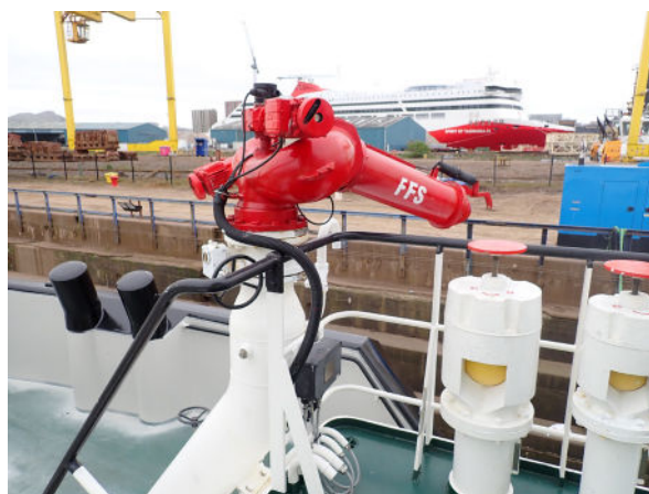
Combined Water & Foam Monitors
